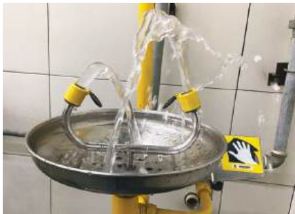
Occasional unbalanced water stream
