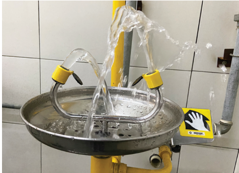
Occasional unbalanced water stream
